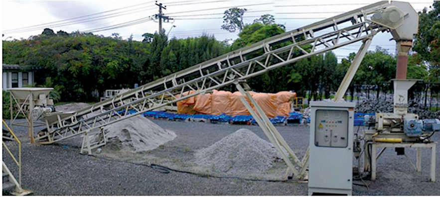
Figure 1 Pilot HPGR facility.
